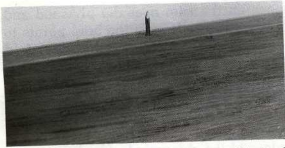
Fig. 1-7. Sand cabinet with care. Close-up view of doublepointed nails. For 1/8-inch edging, let point protrude 1/8 inch.
