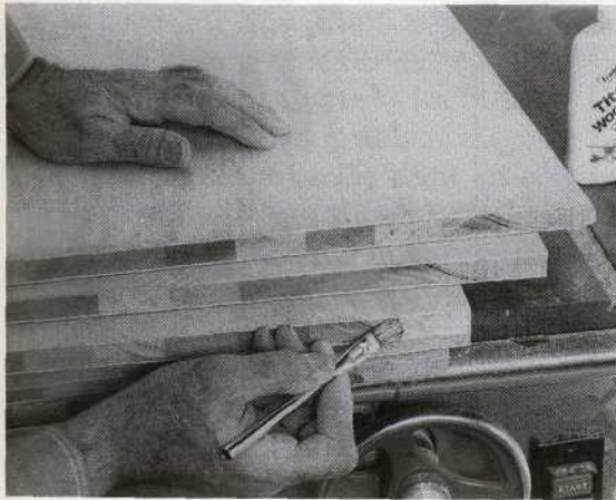
Fig. 1-5. Rough-assemble cabinet parts for fit. Glue sizing the edges of plywood panels with diluted aliphatic resin glue.
