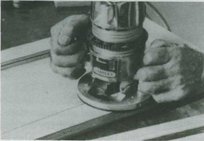
Fig. 24-9. After you've finished assembling the door frames, break the sharp corners with a router fitted with a bevel-trimmer bit.
