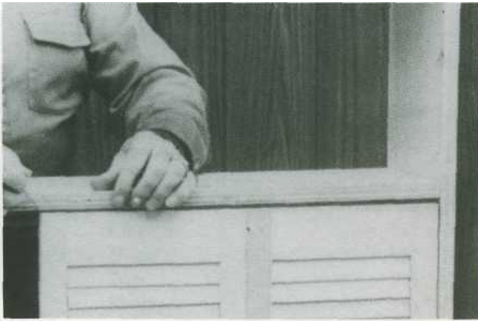
Fig. 22-3. To locate position for dividers, set two doors side by side, make a mark on shelf edge even with door, another mark \frac{3}{16} inch from first indicates inside edge of divider.
